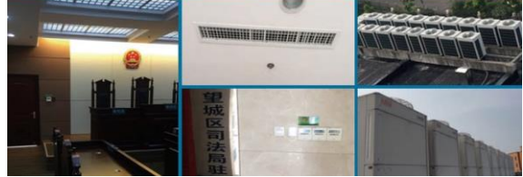
Changsha City People's Court Location : China Completion : 2015 Outdoor unit : 18 Indoor unit : 270
