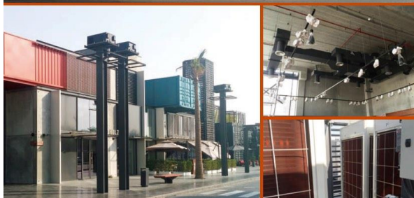
Box Park Al wasl / PK Gulf Location : UAE Completion : 2014 Outdoor unit : 84 Indoor unit : 166
