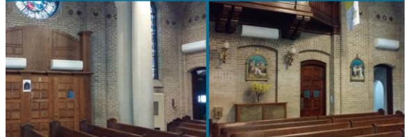
St. Patrick's Catholic Church Location : USA Completion : 2015 Outdoor unit : 2 Indoor unit : 14
